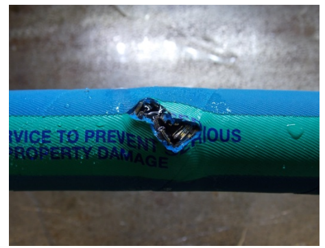
Hose burst close up
